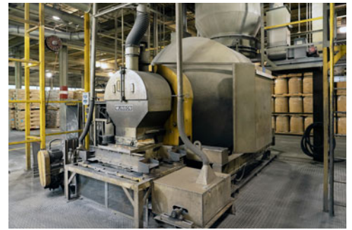
One of two Munson Rotary Batch Mixers, model 700-TSC-180-MS, installed at PLENCO in 1983.
